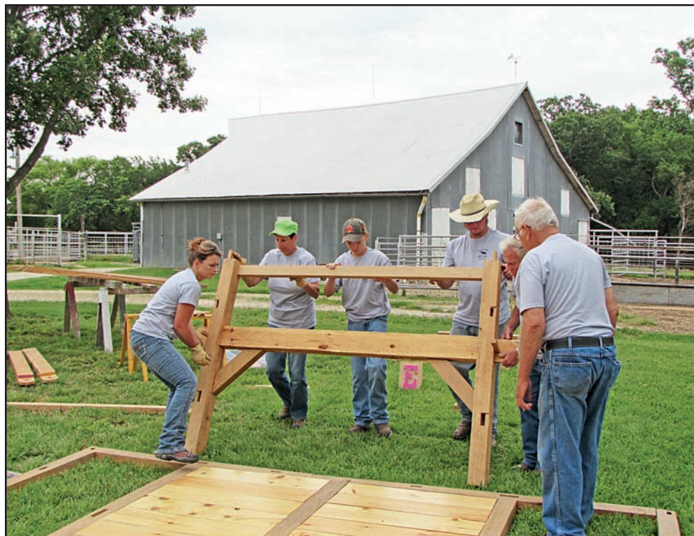
The "A-Team" crew raises the end wall of the timbers scale barn.
